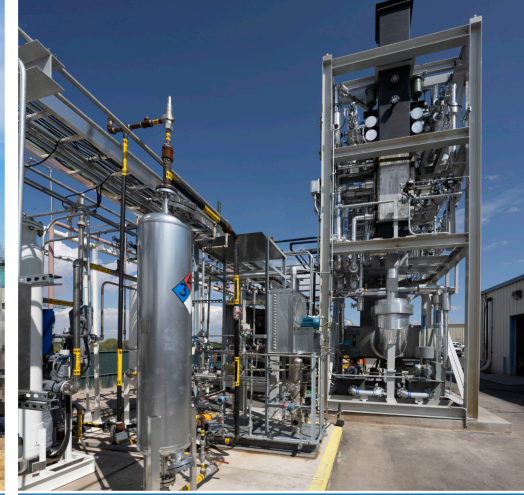
▶ ONSITE HYDROGEN PRODUCTION
